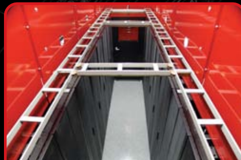
4 layers of heat aisle adjustable cable management
