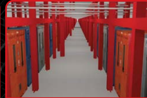
10-10 MVA power rooms empty into the SuperNAPs 1,145 ft long Power Spine
