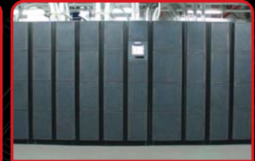
2 x 1.4 MVA grey UPS systems per power room - 84 MVA total at the SuperNAP
