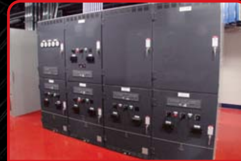
10 x separate grey gateway Switch Gear modules from 12,470 KVA power rooms
