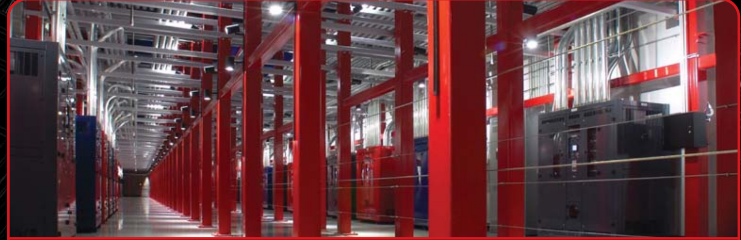
WDMD | Power Spine - The Switch Power Delivery Stanchions
