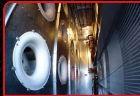
Multiple condensors - System+System +System efficiency chambers
