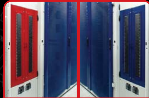
Dual client breaker panels are built into each t-scif cage for added safety
