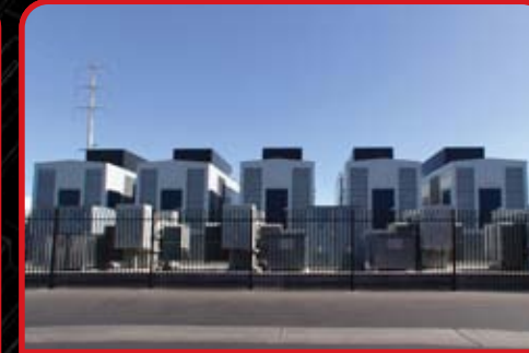
5 x 2.8 MVA Generators for each 10 MVA power room - 50 total at the SuperNAP
