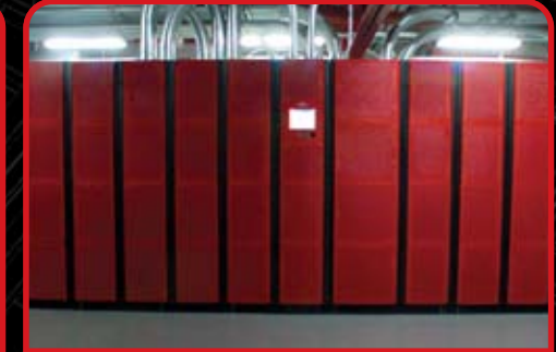
2 x 1.4 MVA red UPS systems per power room - 84 MVA total at the SuperNAP
