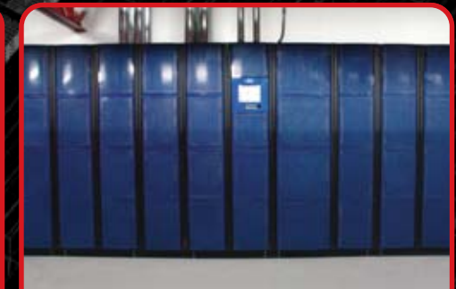
2 x 1.4 MVA blue UPS systems per power room - 84 MVA total at the SuperNAP
