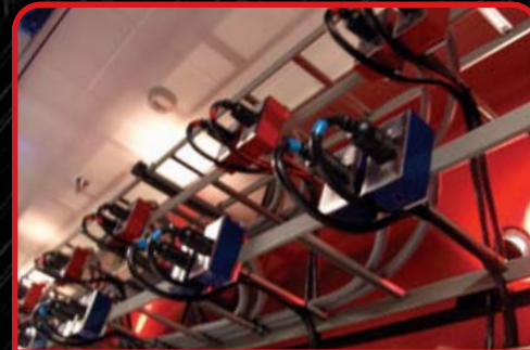
Dual power systems delivered to every cabinet providing 100% up-time
