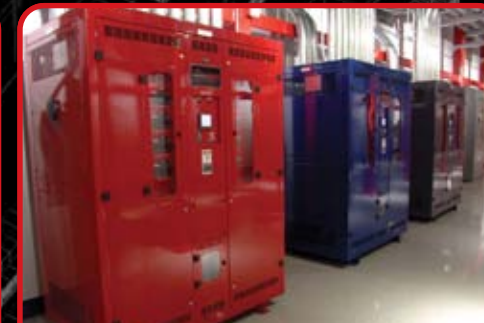
Tri-redundant power systems allow for forever maintainable 100% up-time
