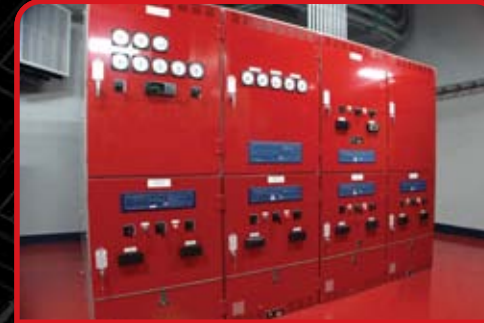
10 x separate red gateway Switch Gear modules from 12,470 KVA power rooms
