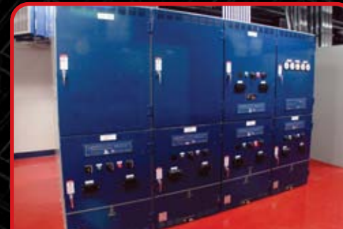
10 x separate blue gateway Switch Gear modules from 12,470 KVA power rooms
